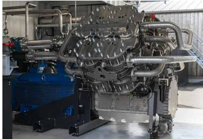
Fig. 1. HoegTemp heat pump prototype installed in Enerin’s test cell
